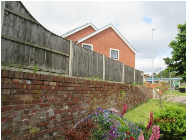
Retaining wall to car park of Flewitt House, taken from the grounds of the resource centre
